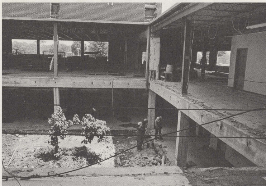
Here's a back view of the SUB/Ely renovation. The new atrium will be located in the open area.
