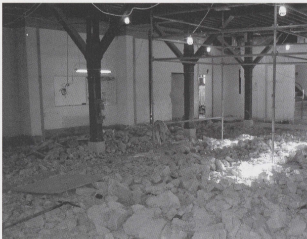
The old cement floor where the swimming pool used to be became debris.
