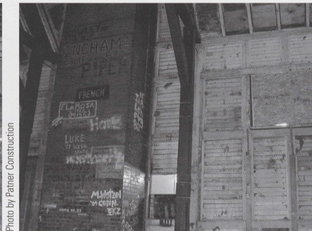
Interior wood slats that were no longer good were removed from the wall next to the well known chimney.
