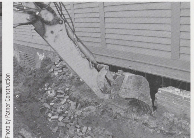
A backhoe went to work removing bricks from the north side of the building.
