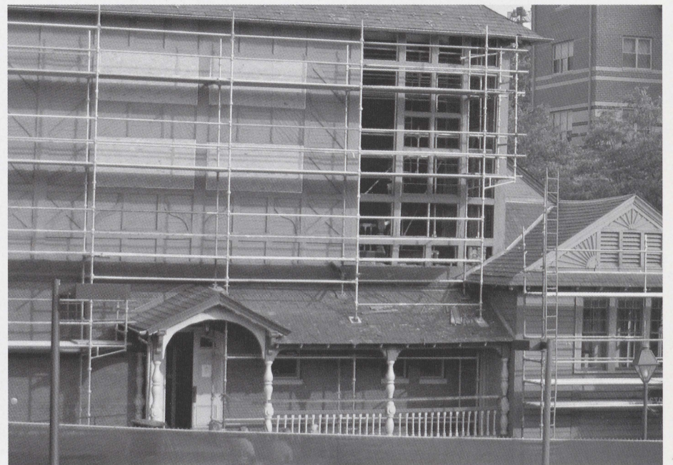
Wood panels were removed from the exterior wall in the northeast corner of “Ole Jim.”
