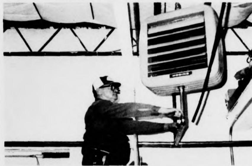
Mr. Charles Brandt, OSD maintenance department, put the final touches on the heater in the new auto maintenance shop.
