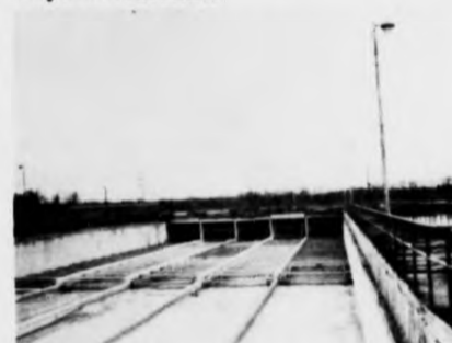
This filtering tank was drained for repairs. The men removed the sand and gravel too.
