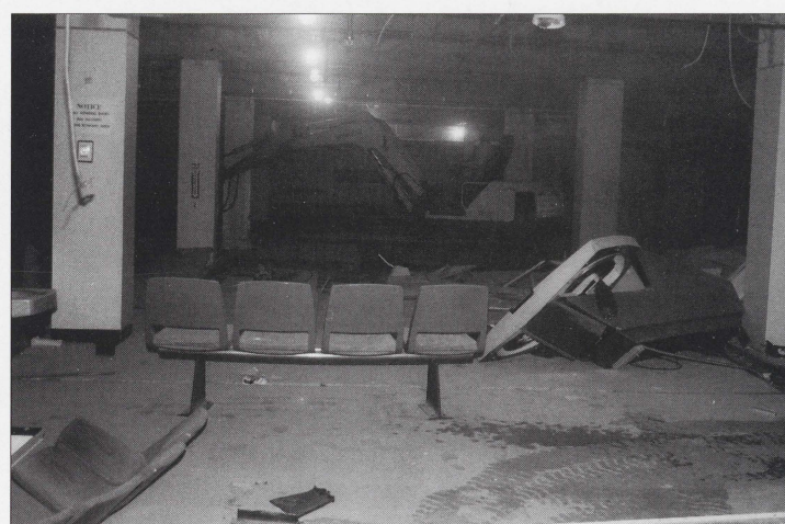
Construction crews remove debris from the lower level of the Student Union Building. The ball returns from the old bowling lanes in the downstairs recreation center are one of the few traces that remain of the former Student Union.
